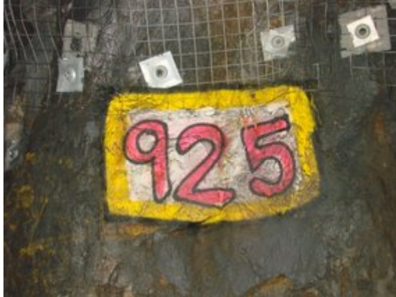
The Anzac Day rockfall occurred on level 925. (ABC News: Jacqui Street)
