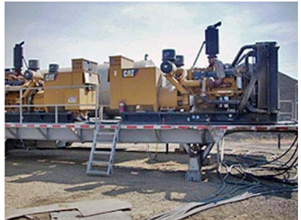
A photo from the federal investigation into James Hussey's death shows the site of the accident. Photo courtesy MSHA
