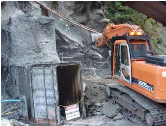
An excavator removes gravel and shotcrete from the seal at the Pike River mine. Photo / supplied
