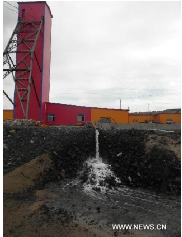
Pumping operation is underway in Lasengzhong Changfu Coal Mine in the Hainan District of Wuhai, north China's Inner Mongolia Autonomous Region, Aug. 20, 2011. The flooding occurred at about 4:30 p.m. Friday at the Lasengzhong Changfu Coal Mine.
