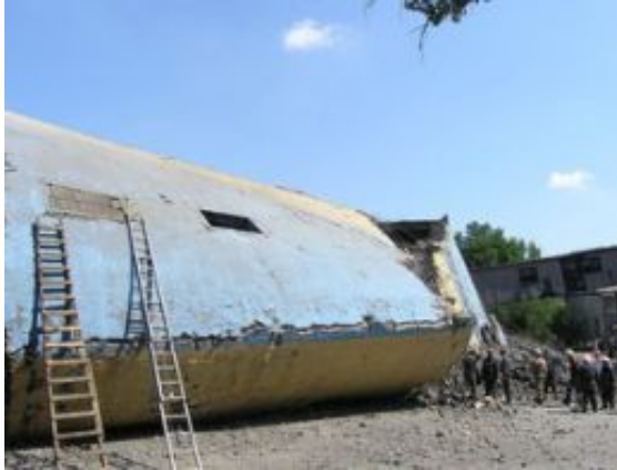
The restoration of the Bazhanov mine in Donetsk Region will take sixteen months in the wake of the July 29 accident that claimed eleven lives.
