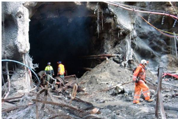
Photograph taken during the removal of the portal seal at the Pike River Mine.
