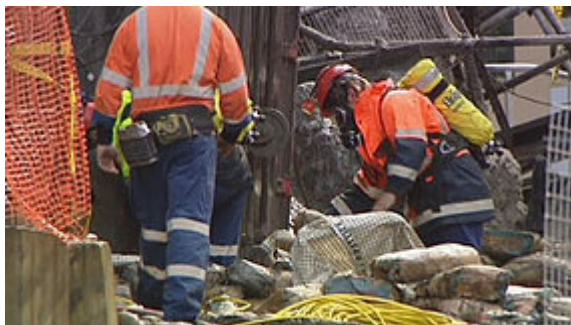
Rescue workers wearing breathing apparatus entered the main tunnel this morning. (TV NZ)
