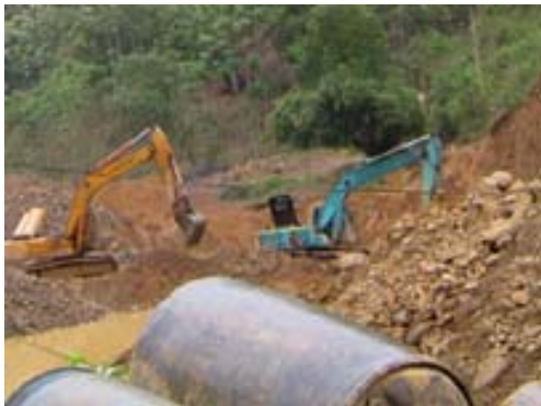
The site of a gold mine collapse that killed five in the central province of Nghe An Sunday
