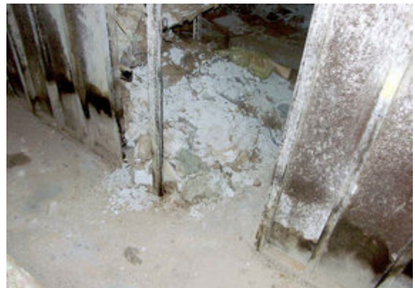
Broken bags of asbestos lie in an abandoned mine (NSW Ombudsman)
