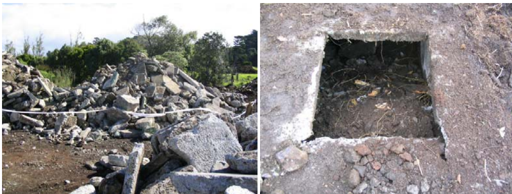
Figure 11: Contaminated concrete ready to be carted to landfill and one of the in ground CCA holding tanks uncovered.
