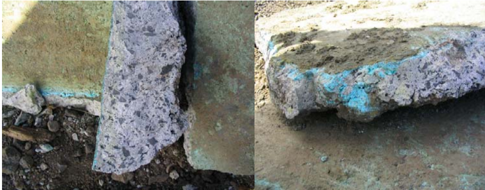
Figure 12: Some of visible signs of Copper contamination in the concrete from the sawmill drip pad.
