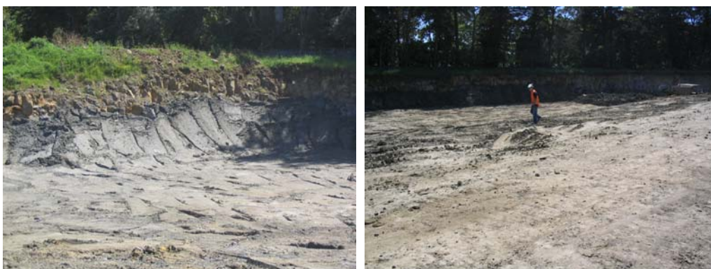
Figure 13: The clay cell which was constructed on site to contain mildly contaminated material.
