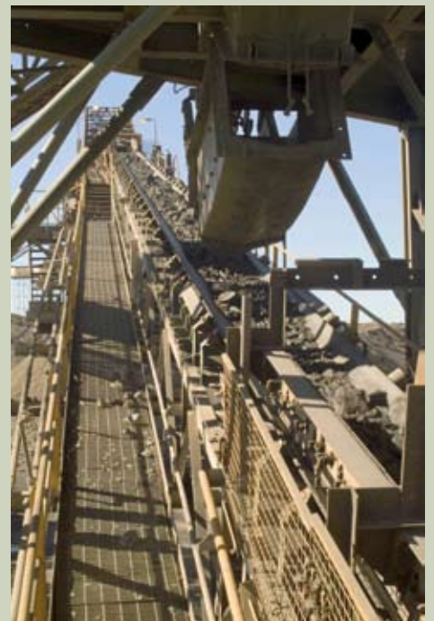
Isolating energy sources to moving machinery, such as conveyors, are essential before work on the plant is undertaken.
