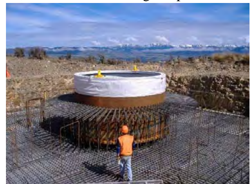
Photo of foundations prior to pouring, showing the huge quantities of steel reinforcing
